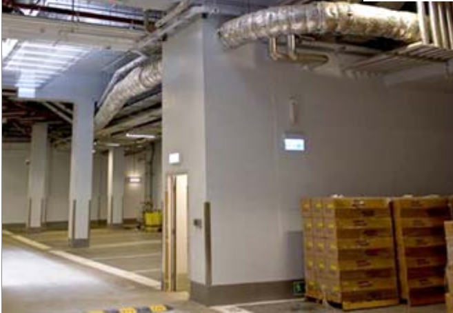
Solar chimney in the basement carpark
