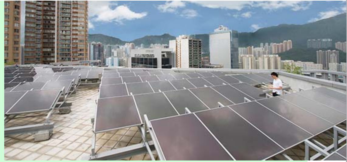
View of photovoltaic panel on upper roof
