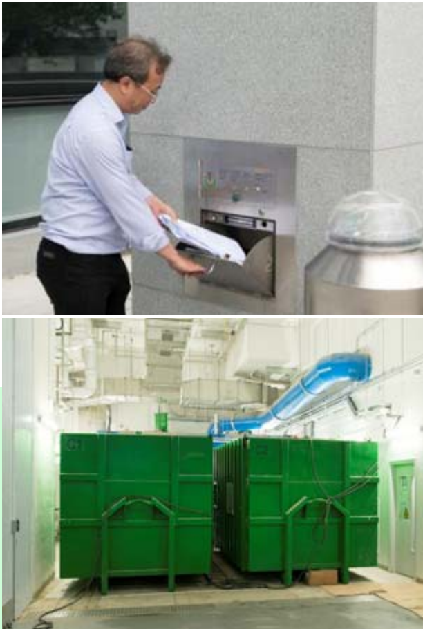
Refuse disposal inlets for paper and general waste are installed in each floor and inlet for general waste on Ground Floor (top) and a central refuse collection station (bottom) is set at the basement
