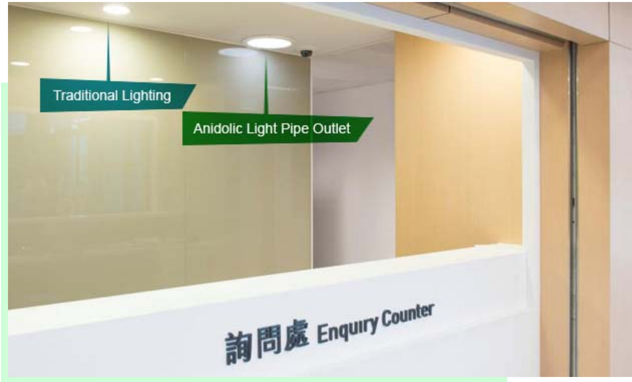
Anidolic light pipe in the Building Management Office providing similar luminosity to traditional lighting
