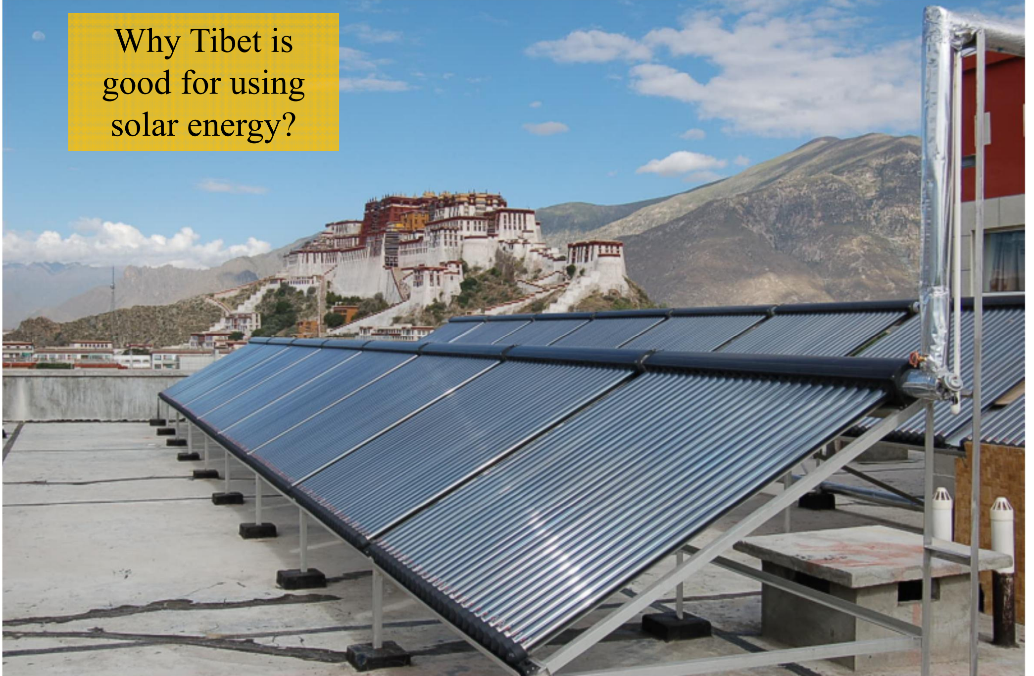
Evacuated-tube solar hot water system in a hotel in Lhasa, Tibet (photo taken by Dr Sam C M Hui)
