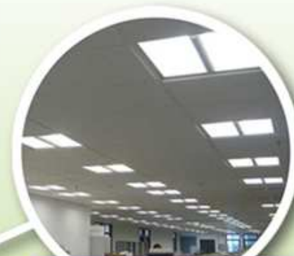
照明裝置 Lighting installation
