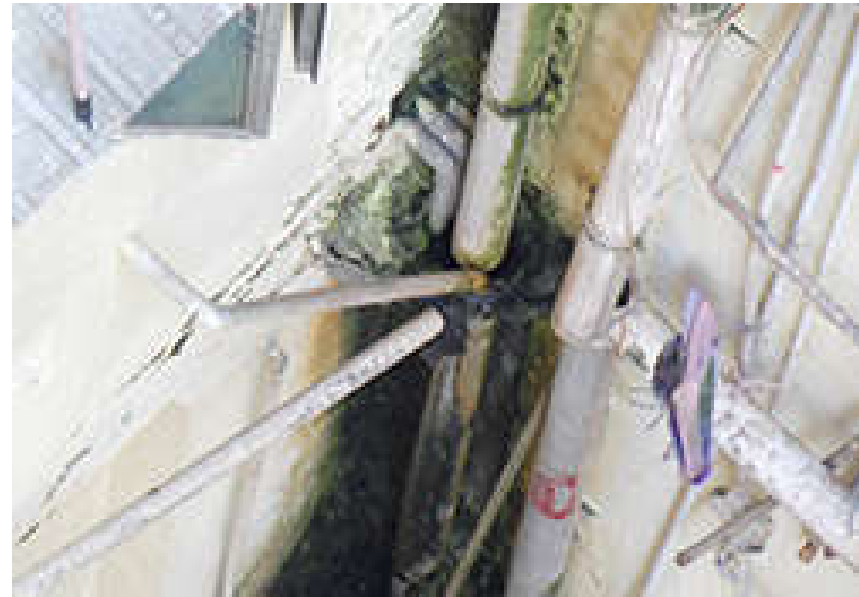
Unauthorised alteration of drainage system
