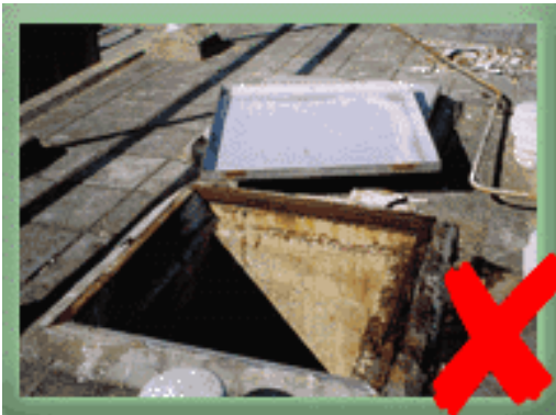
Damaged water tank cover
