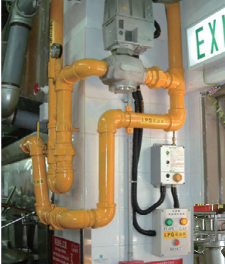
Control valve & meter
