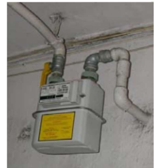
Figure 3: An installation pipe and gas fittings
