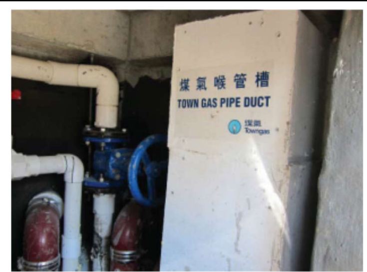
A town gas pipe duct
