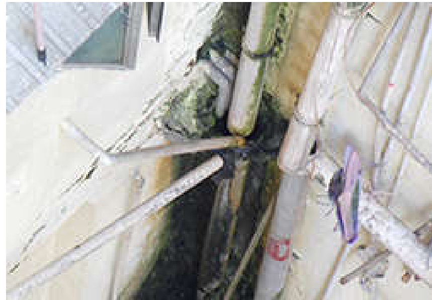
Unauthorised alteration of drainage system
