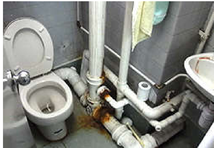
Rusty internal drainage pipes
