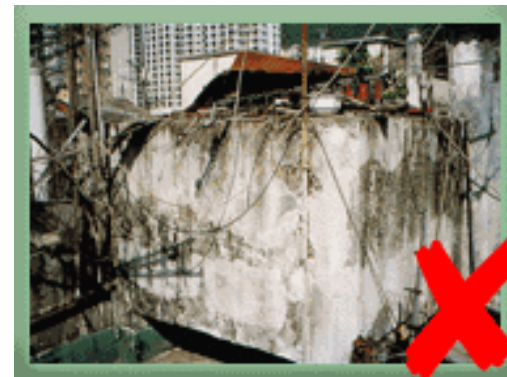
Storage tank without proper maintenance & management
