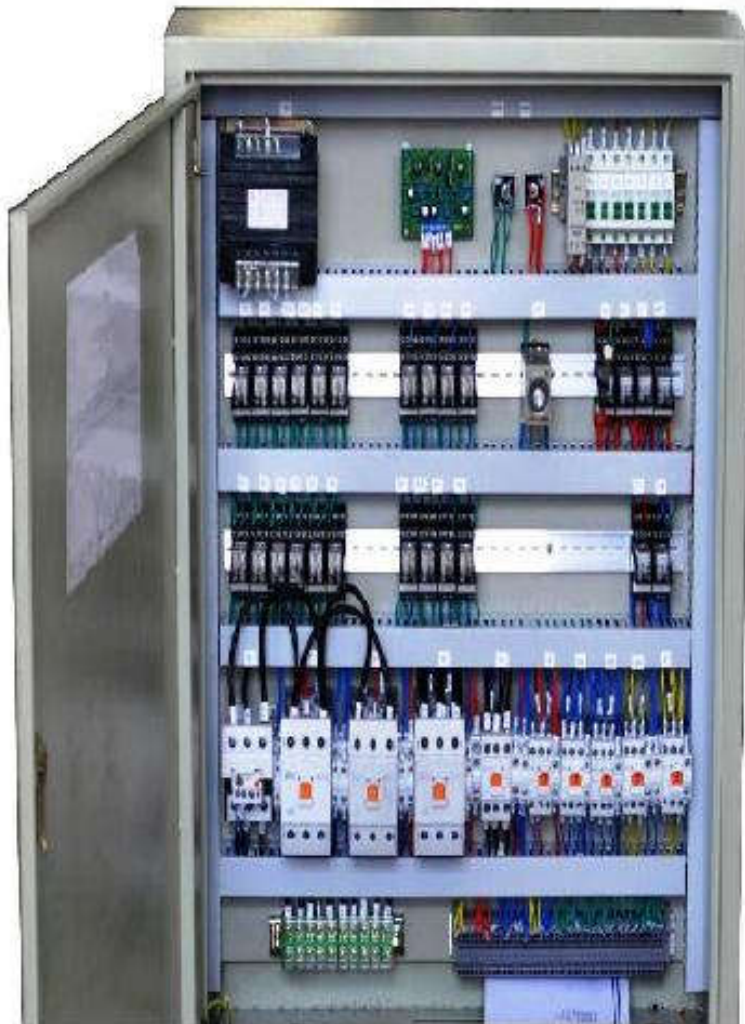
Relay based controller
