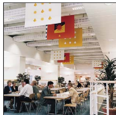
Fig 2 Public place with emergency lighting
