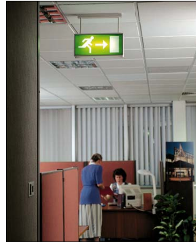
Fig 1 Office with emergency lighting
