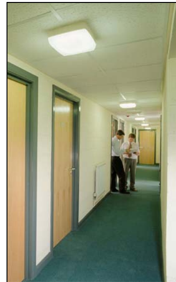
Fig 38 Panther luminaires on escape route
