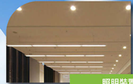
照明裝置 Lighting installation
