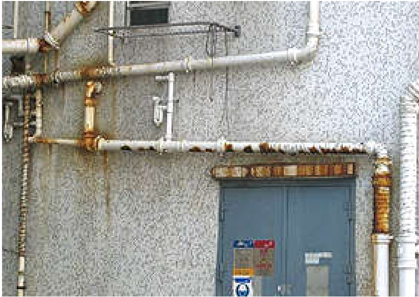
Rusty external drainage pipes
