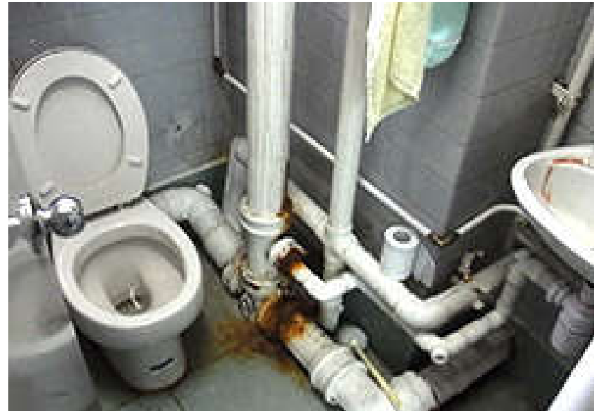
Rusty internal drainage pipes
