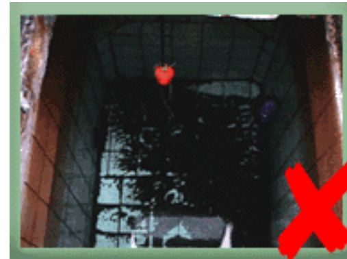
Water tank not cleaned
