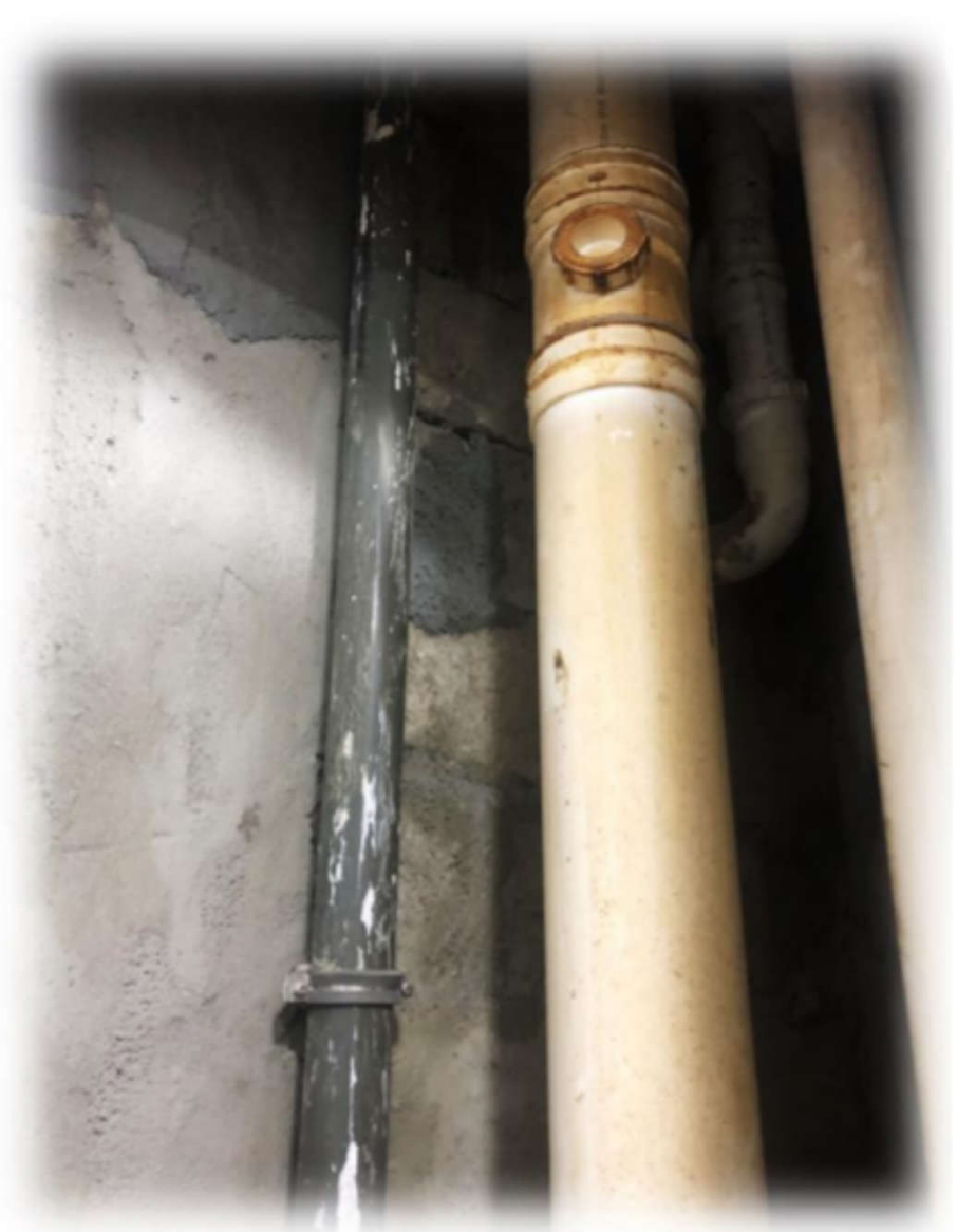
Internal pipe duct accessible from common parts
