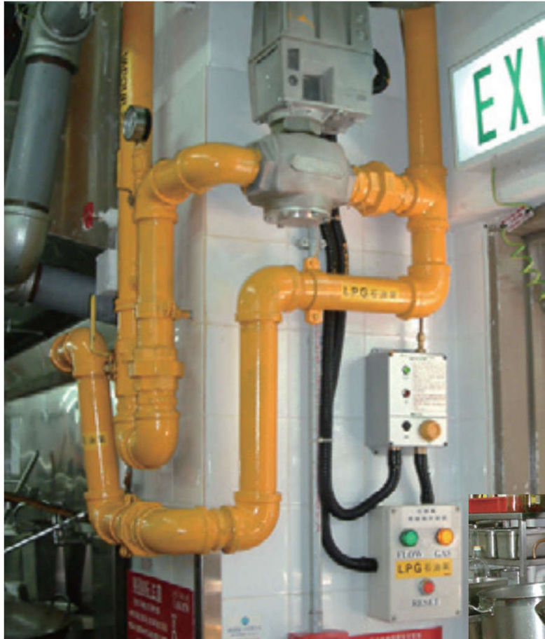
Control valve & meter
