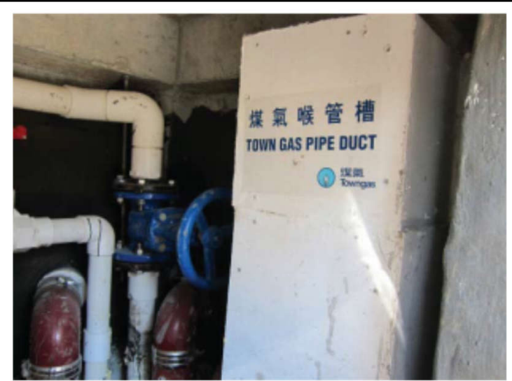
A town gas pipe duct
