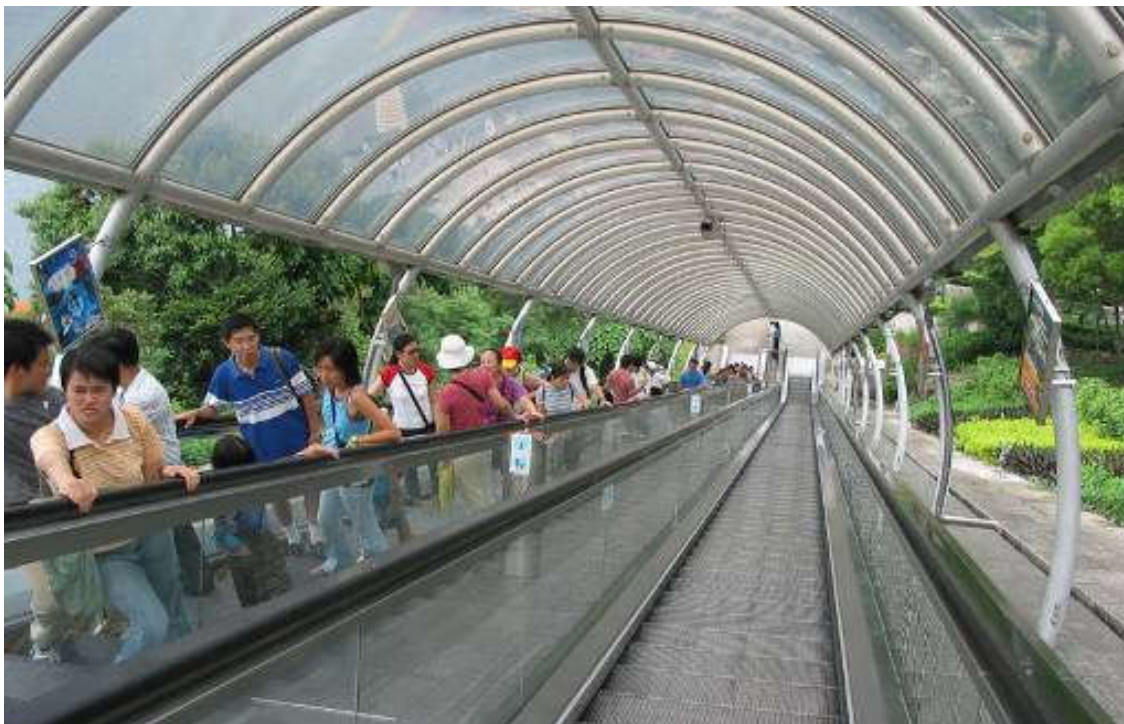
Ocean Park (longest outdoor escalator, total 220 m)
