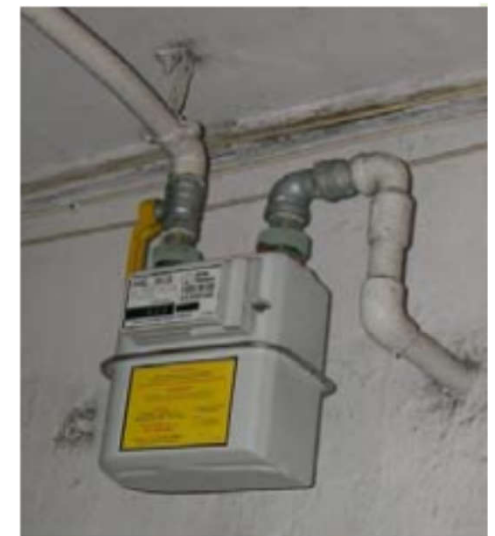
Figure 3: An installation pipe and gas fittings
