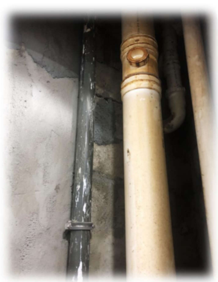
Internal pipe duct accessible from common parts
