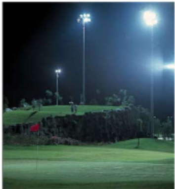
Golf course lighting
