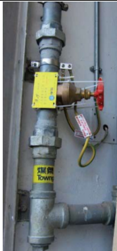
A service valve
