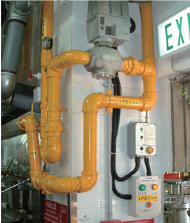
Control valve & meter
