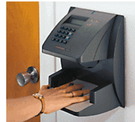
Access Control Terminal
