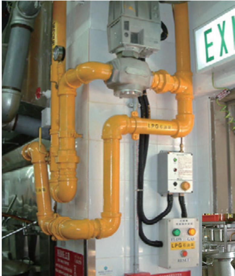
Control valve & meter
