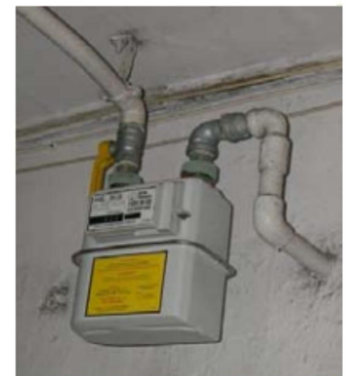
Figure 3: An installation pipe and gas fittings
