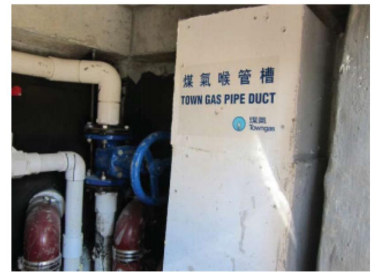
A town gas pipe duct
