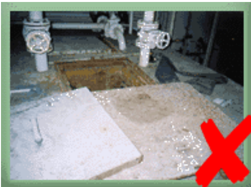
Rusty water tank cover
