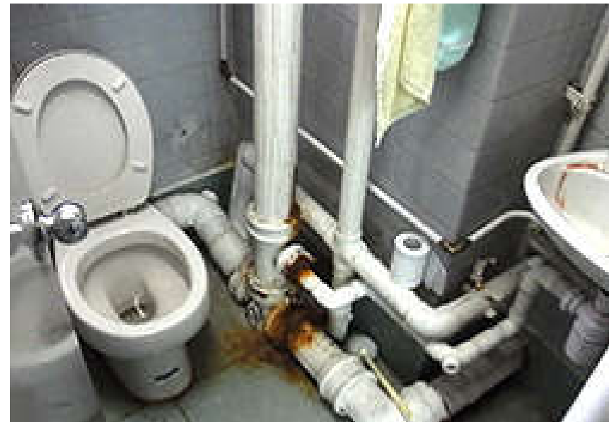
Rusty internal drainage pipes
