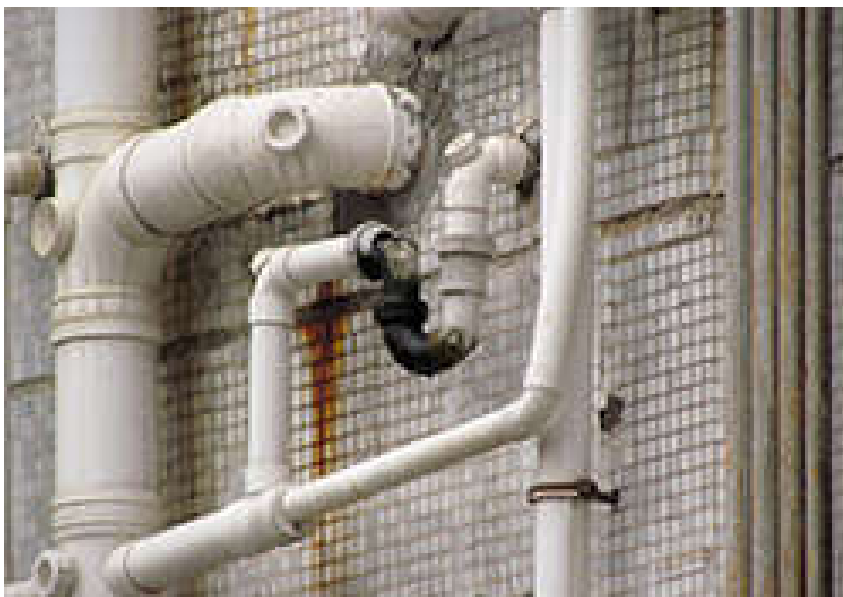
Leaking or broken drainage pipes at external wall
