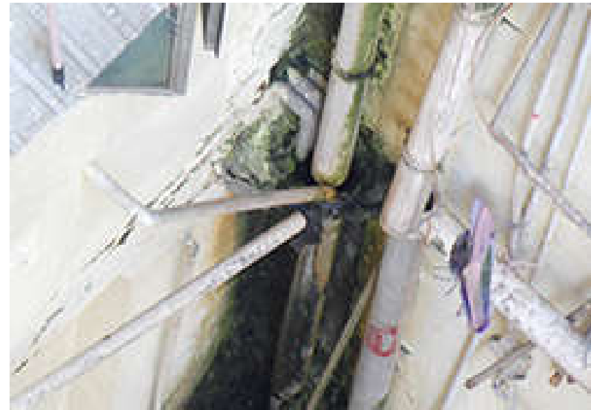
Unauthorised alteration of drainage system
