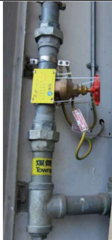
A service valve
