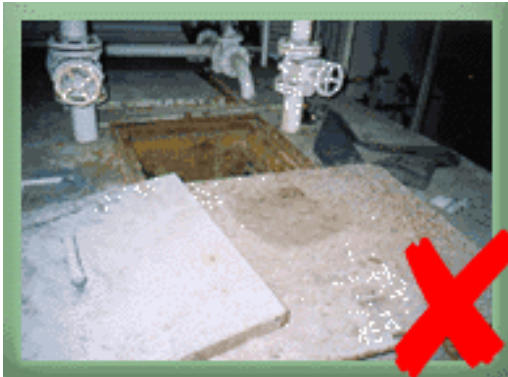
Rusty water tank cover
