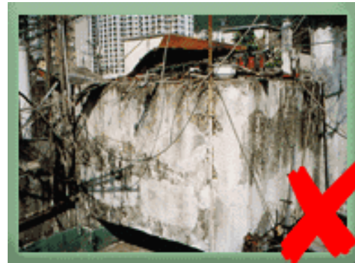
Storage tank without proper maintenance & management
