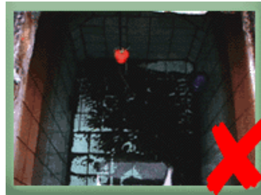
Water tank not cleaned
