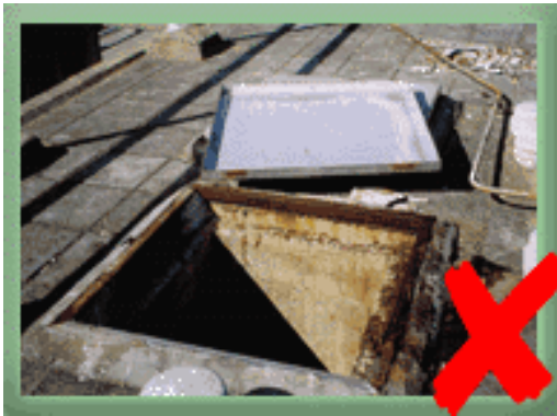
Damaged water tank cover
