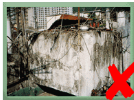
Storage tank without proper maintenance & management
