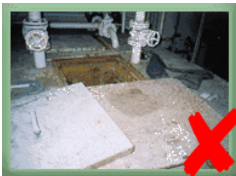
Rusty water tank cover
