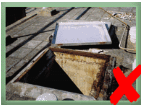
Damaged water tank cover
