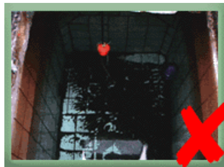
Water tank not cleaned
