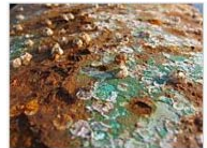
Corrosion caused partly by barnacles
