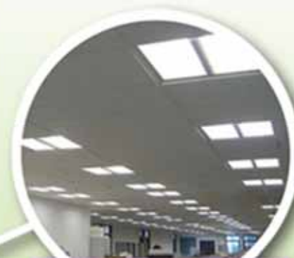
照明裝置 Lighting installation
