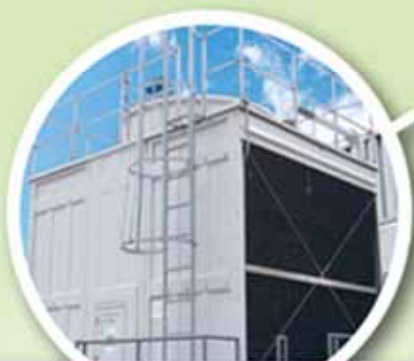
空調裝置 Air-conditioning installation
