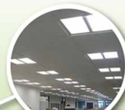
照明裝置 Lighting installation
