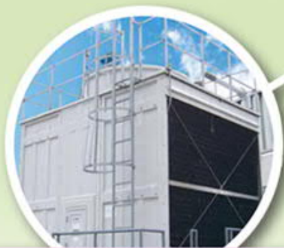
空調裝置 Air-conditioning installation
