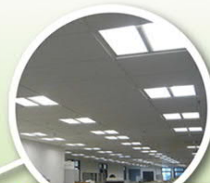
照明裝置 Lighting installation
