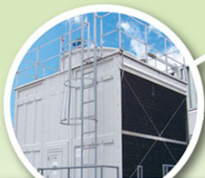
空調裝置 Air-conditioning installation
