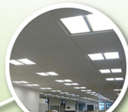
照明裝置 Lighting installation
