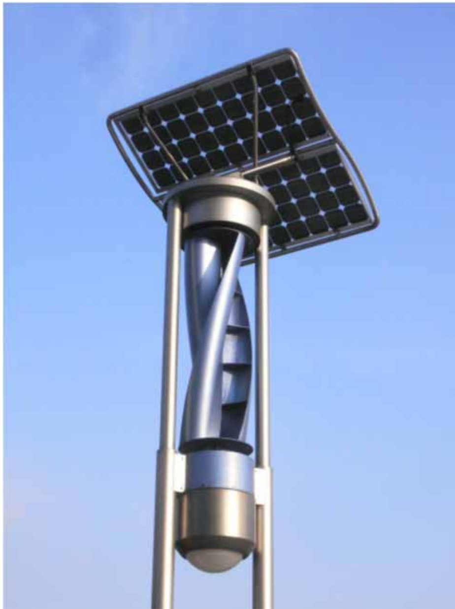
PV-wind lamp pole (installed at HKU Faculty of Medicine Building)
