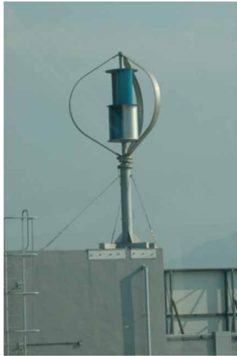
1.5 kW vertical wind turbine (installed at EMSD Headquarters)
