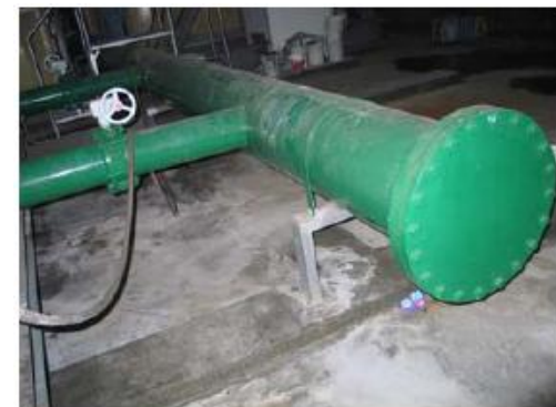
A long dead leg extends from the main pipe
