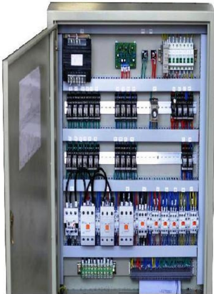
Relay based controller
