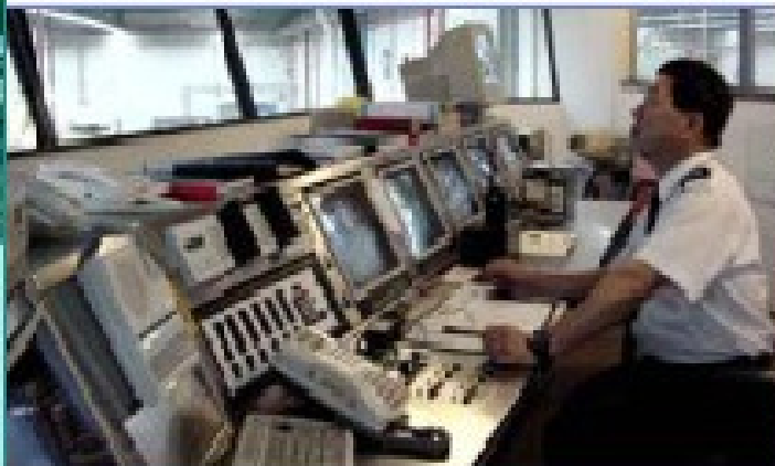
Security control centre
