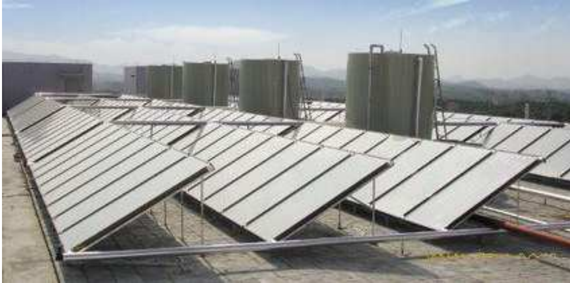
Flat-plate solar collector
