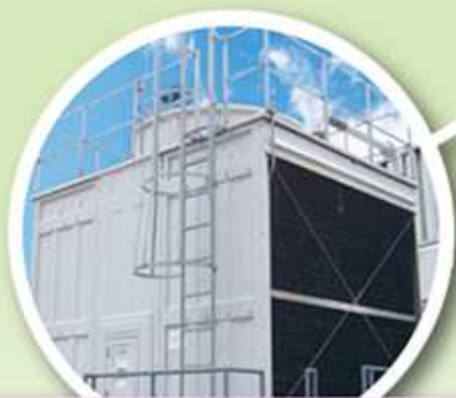
空調裝置 Air-conditioning installation
