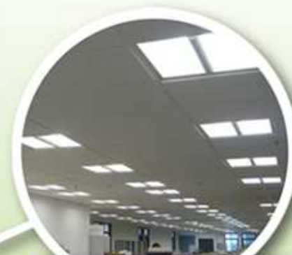
照明裝置 Lighting installation
