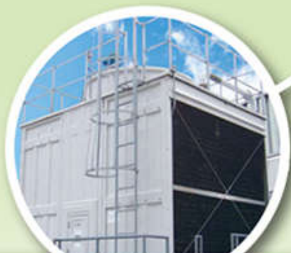
空調裝置 Air-conditioning installation
