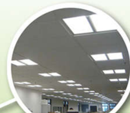
照明裝置 Lighting installation
