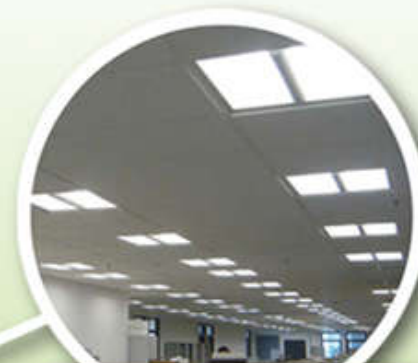
照明裝置 Lighting installation
