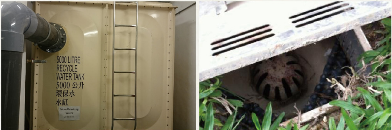
Figure 17 Recycle water tank and a rainwater inlet on the green roof
