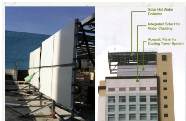
Figure 30 Solar hot water cladding
