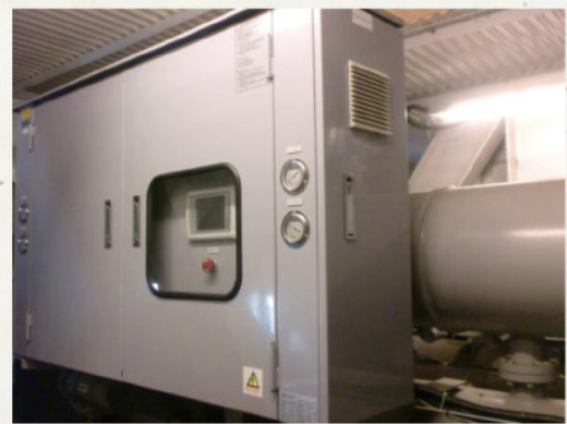
Figure 11 The chiller is controlled by EOS control algorithms
