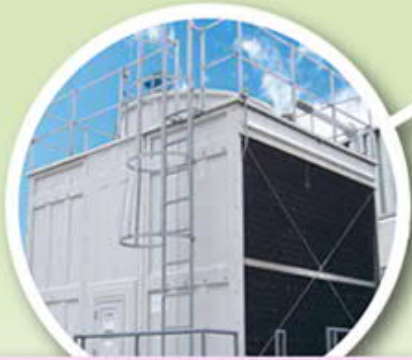
空調裝置 Air-conditioning installation
