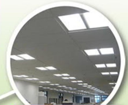
照明裝置 Lighting installation
