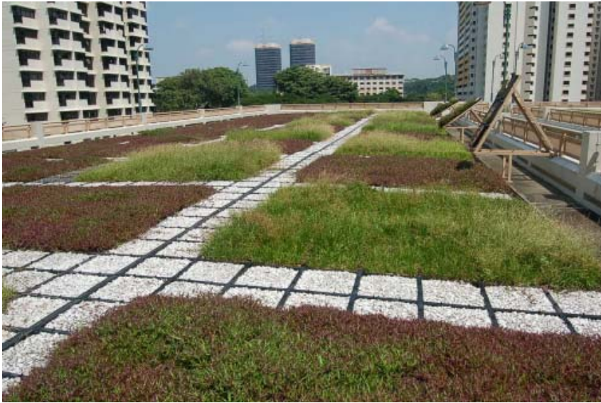
Carpark roof of public housing (modular green roof)
