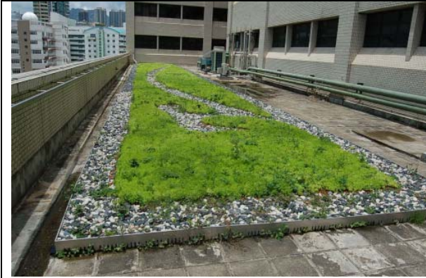
4/F green roof (15 Jul 2009)
