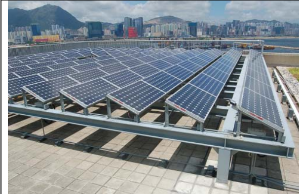
10/F solar PV system (15 Jul 2009)
