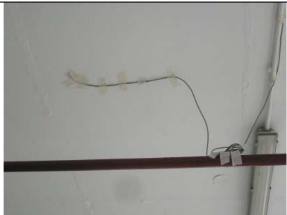
Temperature sensor at carpark ceiling
