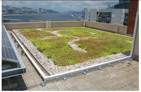
10/F green roof (15 Jul 2009)
