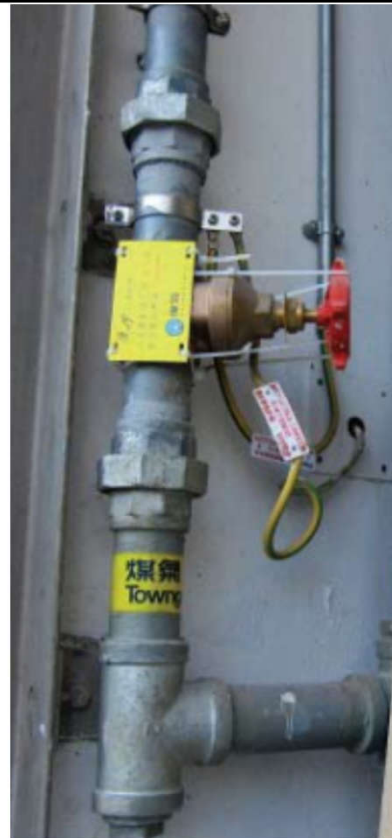
A service valve
