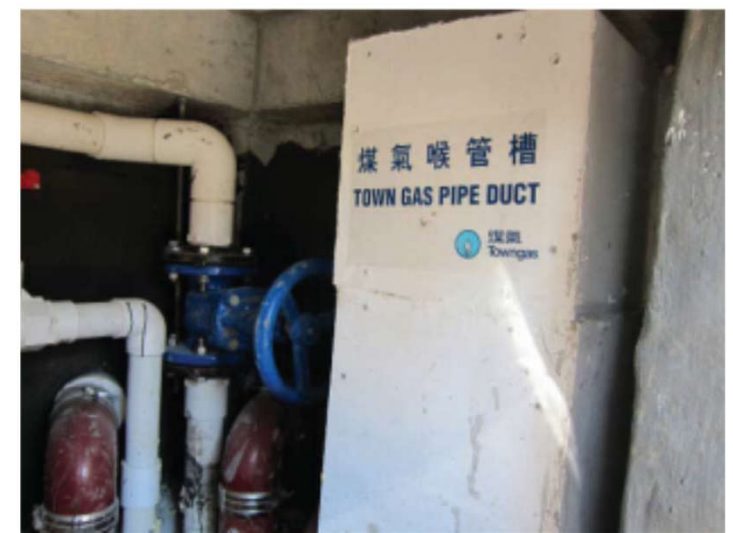
A town gas pipe duct
