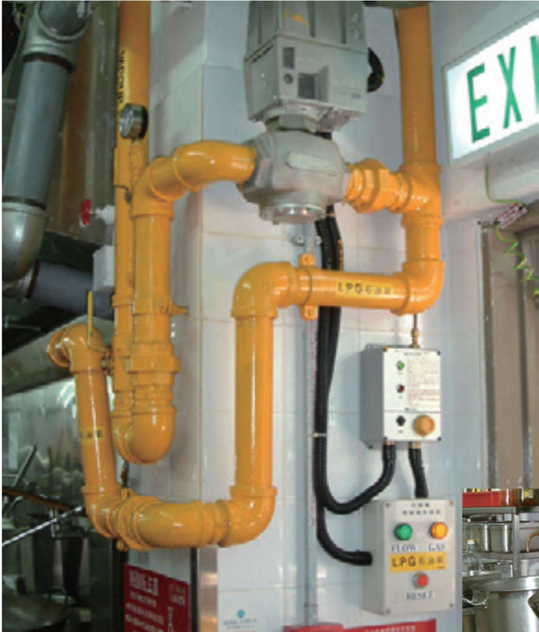
Control valve & meter
